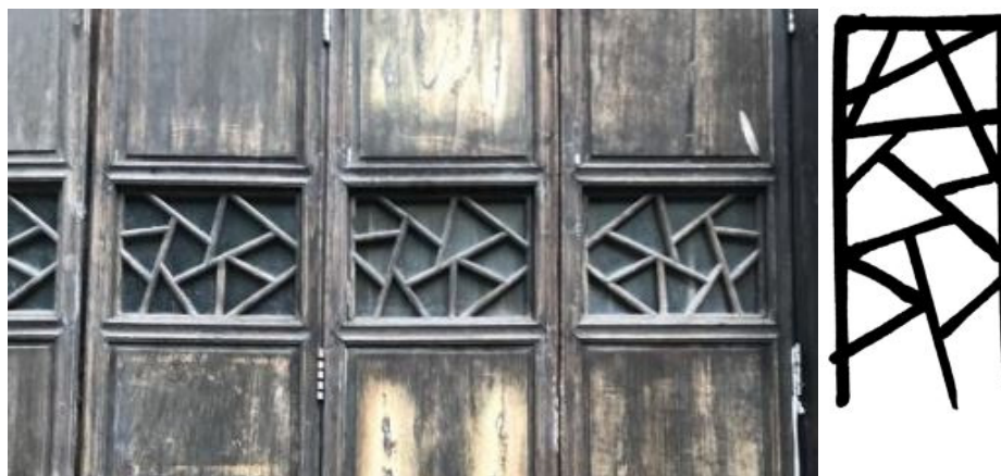
Figure 13. Ice crack on the gate of shanghetang
